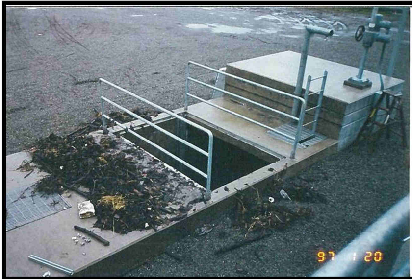
Left: Debris build-up during the larger storms
