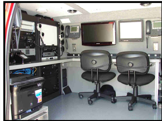
Will contain communications technology to manage critical incidents from remote locations
