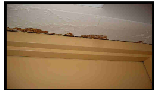
Corrosion around exterior exiting door
