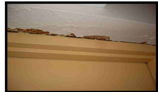
Corrosion around exterior exiting door
