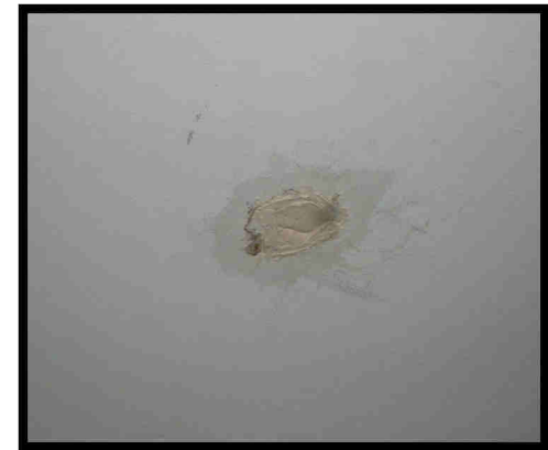
Constant Repairs from Leaking Roof
